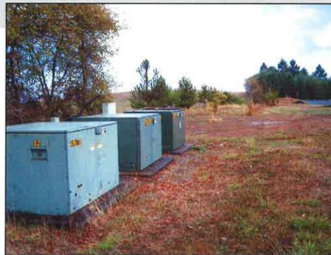
Termination boxes and switches along new underground cable route.
