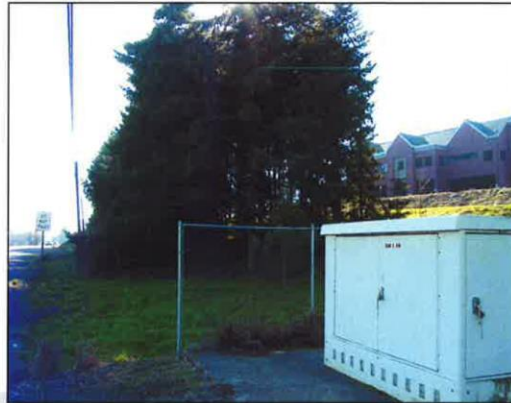
Solution: Converted overhead power source to underground in conduit where only the overhead phone line remains along outside of required tree buffer zone for hospital facility.
